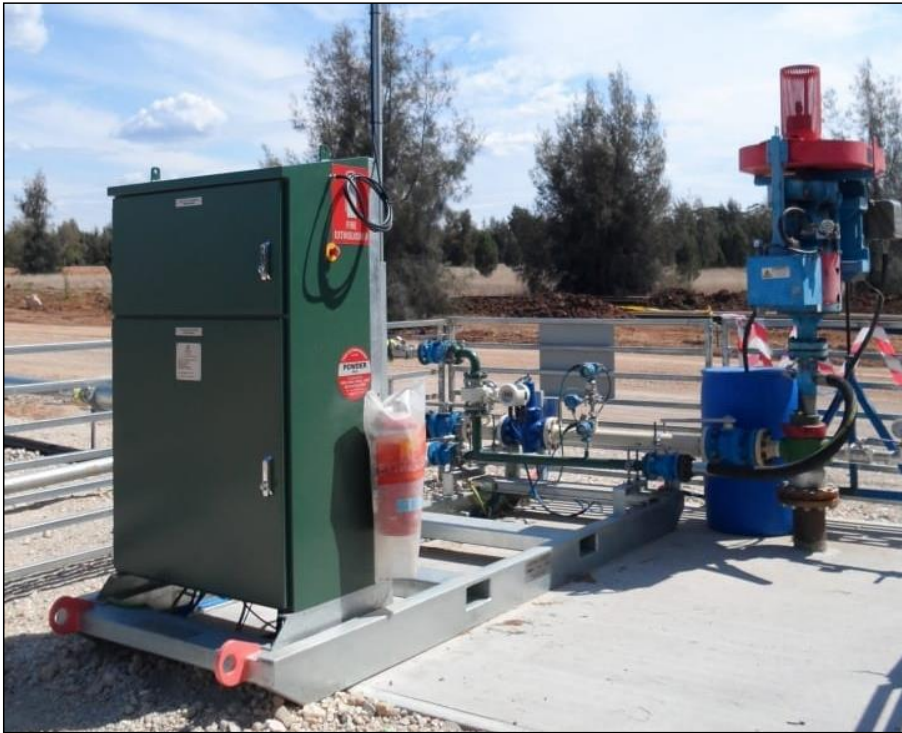
Figure 3.38: Example SIS gas drainage relocatable skid.
