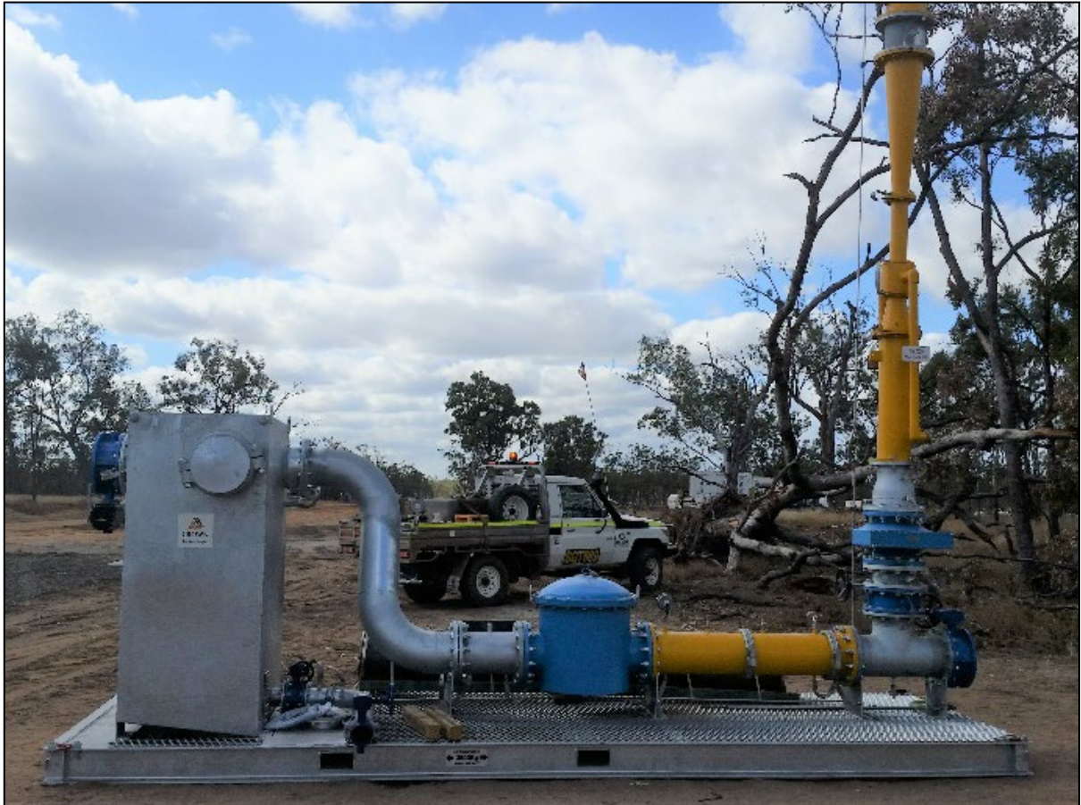
Figure 3.39: Example venturi skid equipment.
