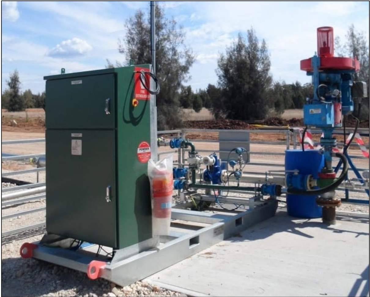
Figure 3.38: Example SIS gas drainage relocatable skid.
