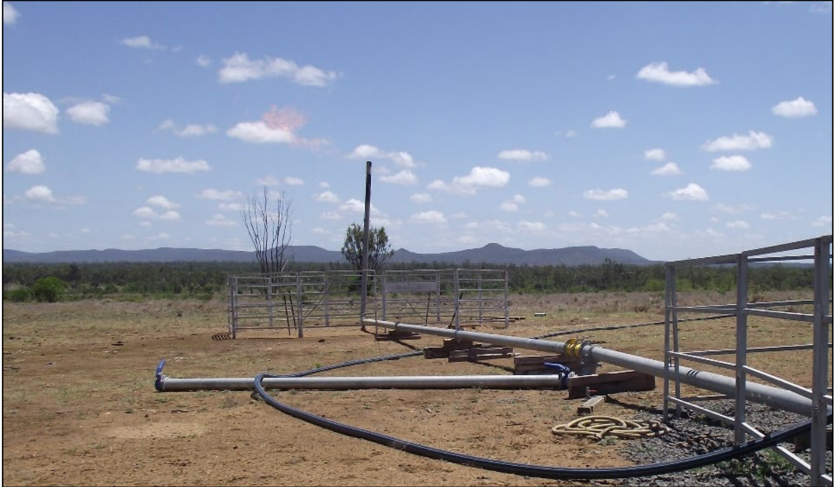
Figure 3.40: Example flare installation.
