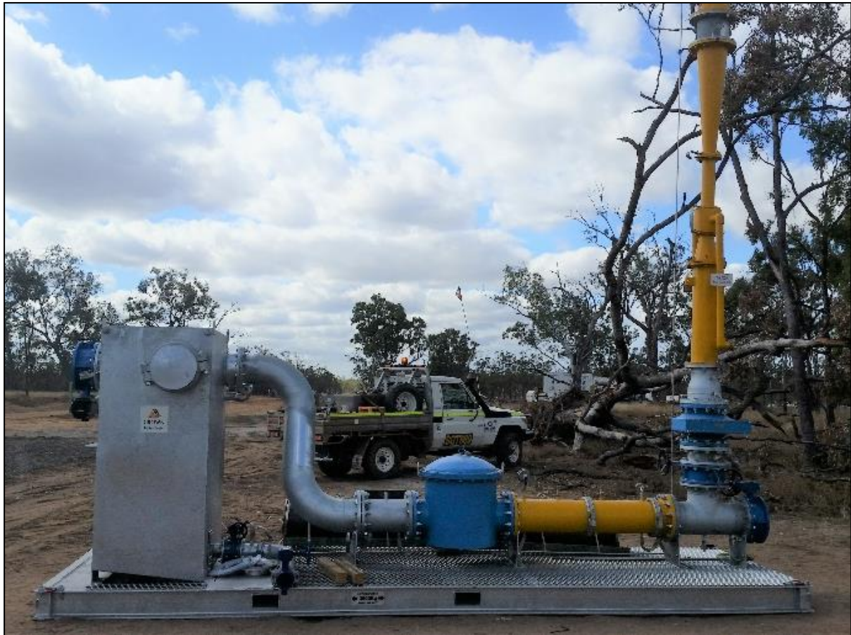
Figure 21.33: Example venturi skid equipment
