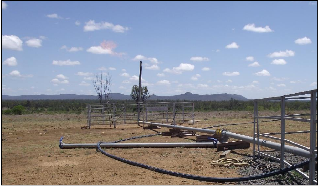
Figure 21.34: Example flare installation
