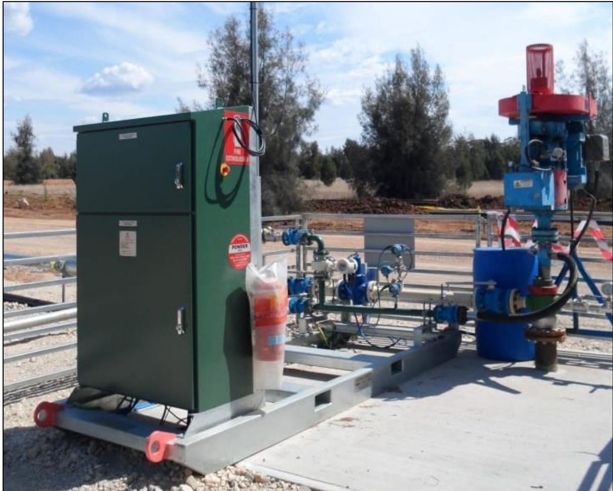
Figure 21.32: Example SIS gas drainage relocatable skid
